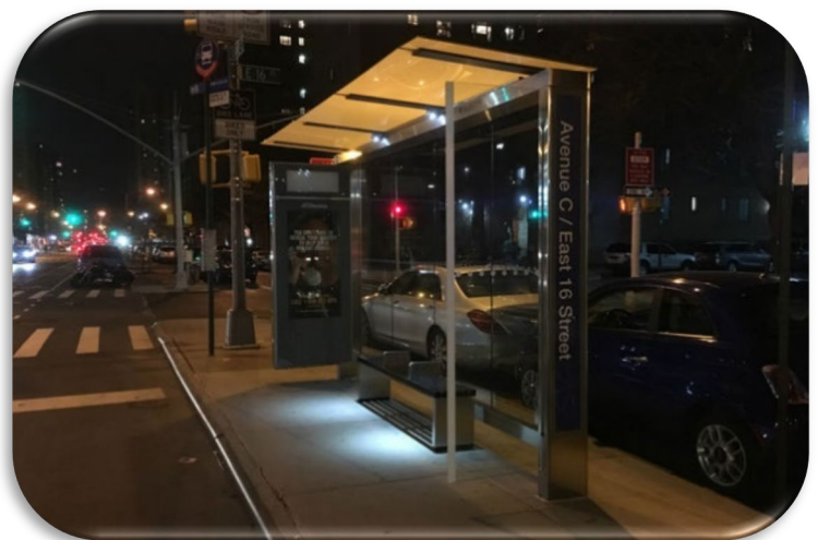
Figure 77. NYC's first solar powered bus shelter installed in 2016.
