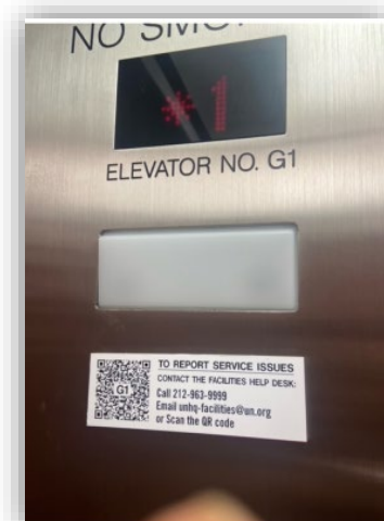
Figure 29. Elevator with QR code.
